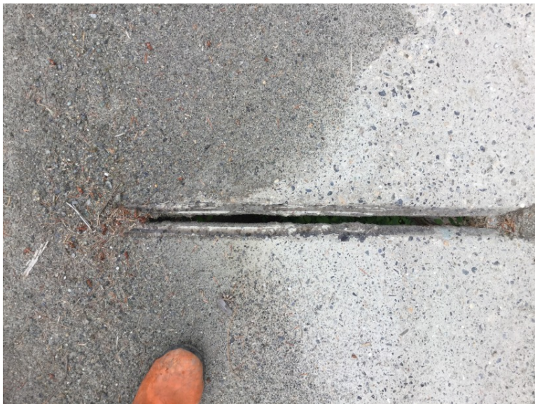
Missing deck joint seals
