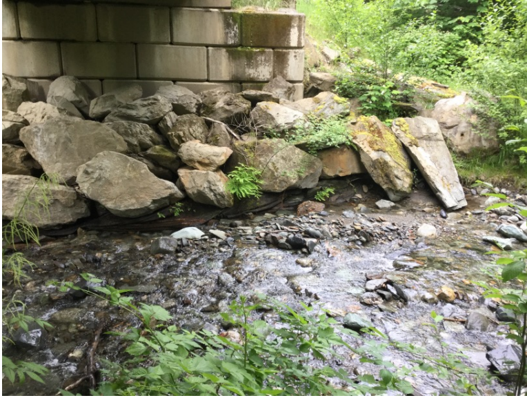
Riprap scour at right bank
