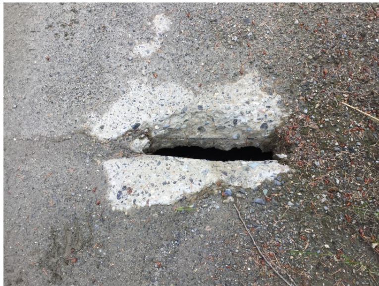
Damage to to ballast wall and deck panel at right approach
