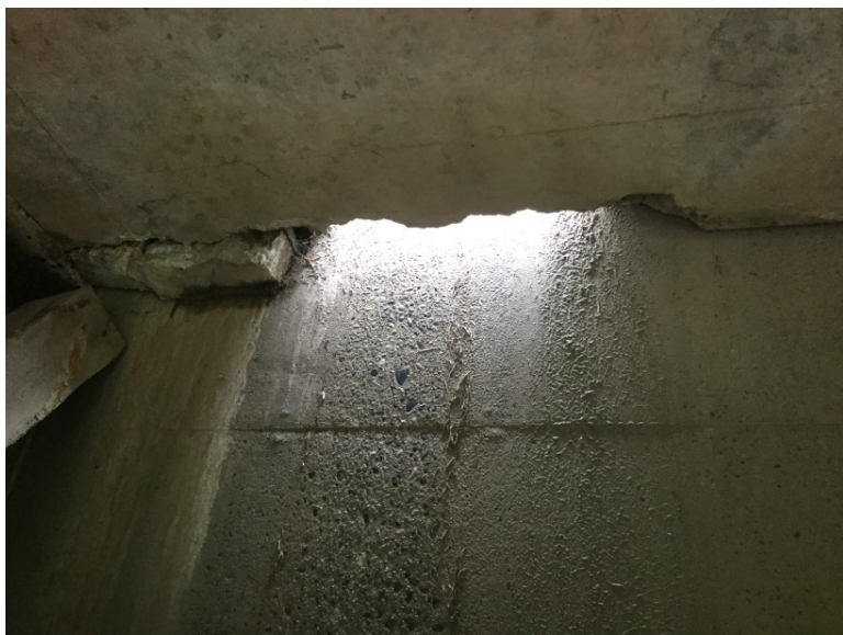
Damage to panel 1 at right approach
