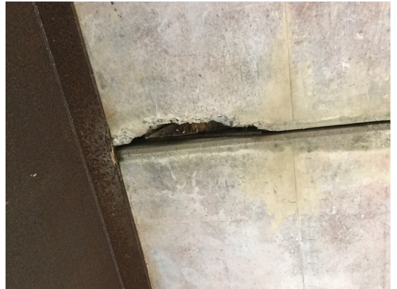
Damage to panel 1 at right approach
